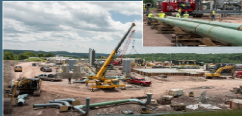
Williams Company, Church Compressor Station
