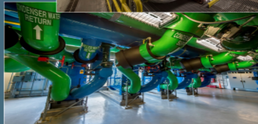
MIT, Boiler & Deaerator
